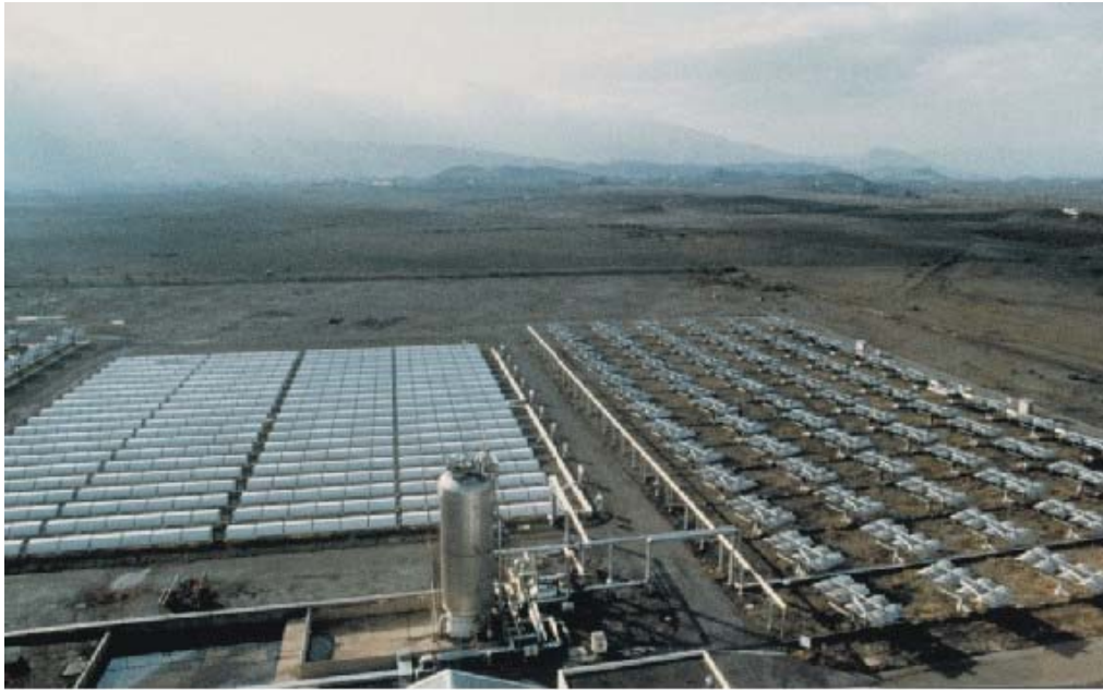
Figure 3. The 500 kW e IEA-SSPS/DCS experimental power plant of the Consortium ACUREX/MAN in Almería (Spain). (Source: PSA)
